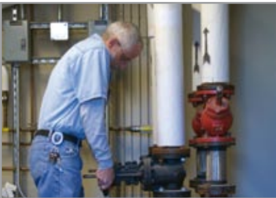
The SpiroVent Superior removed a huge volume of air during the start-up phase, thus enabling very quick commissioning.
