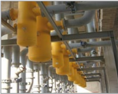
23 SpiroCombis keep the climate conditioning system at Barcelona Airport constantly free of gases and dirt particles.
